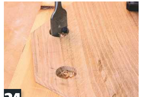
24 Mark hole centres and cramp board to backing material. Bore ends of cutout with 25mm flat bit
